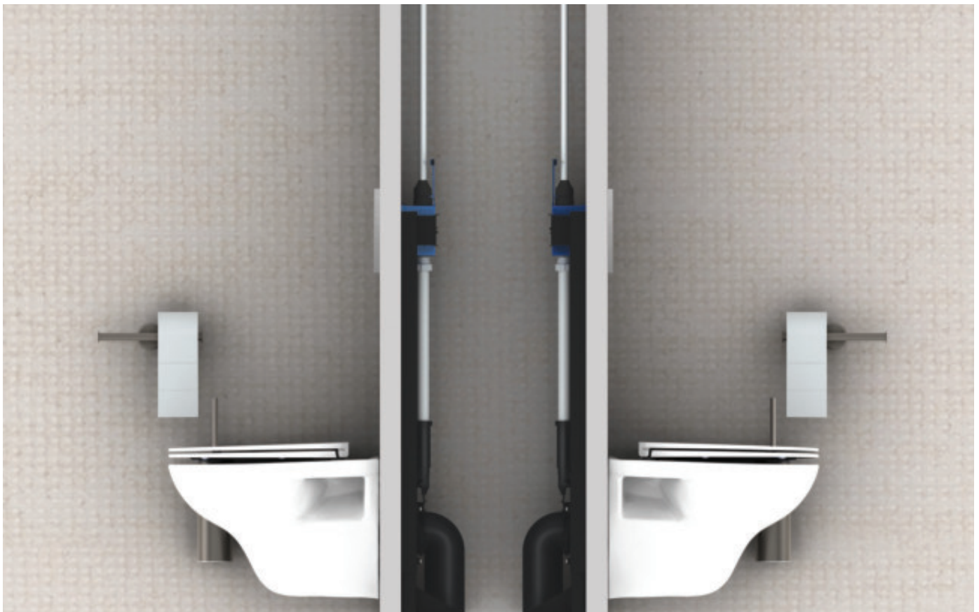
Two TEMPOFIX 3 fire retardant frame systems installed back to back.
